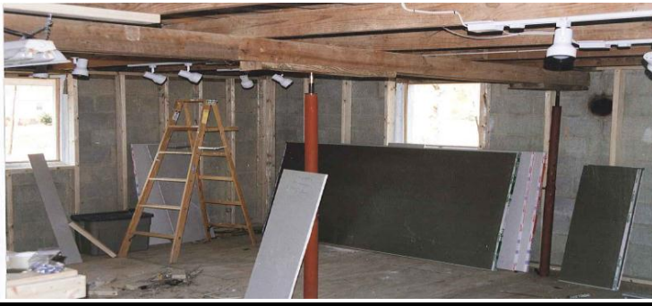
After the floor was in but before the walls and office were built.
