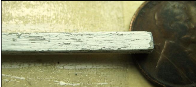
Close up of peeling paint
